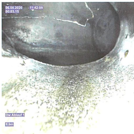
H 01_d83d3b66-658e-4212-8bde-8efd955c4da9_20200807_103 845_099.jpg, 00:00:00, 9.80m Rohrende / Abzweiger
